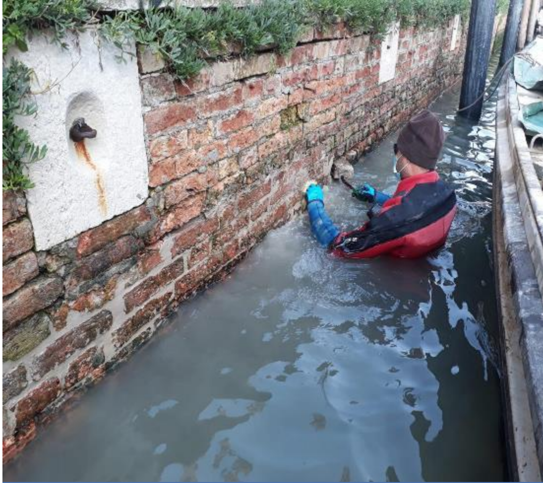
Brick joints underwater
